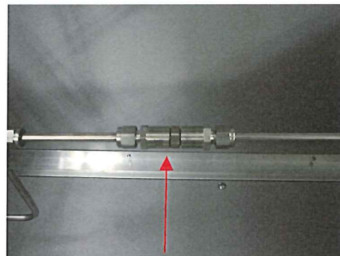
Safety-valve inside the BOX
